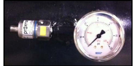
Figure 4: Pressure gauge and transducer
