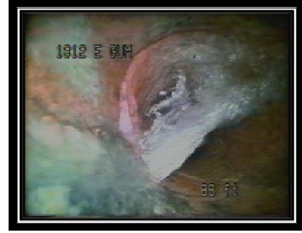
Figure 1: Leaking Lateral Pipe
