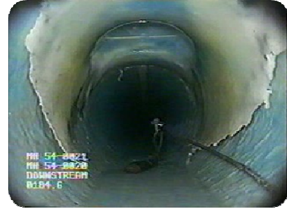
Figure 2: Failed Glued Patch
